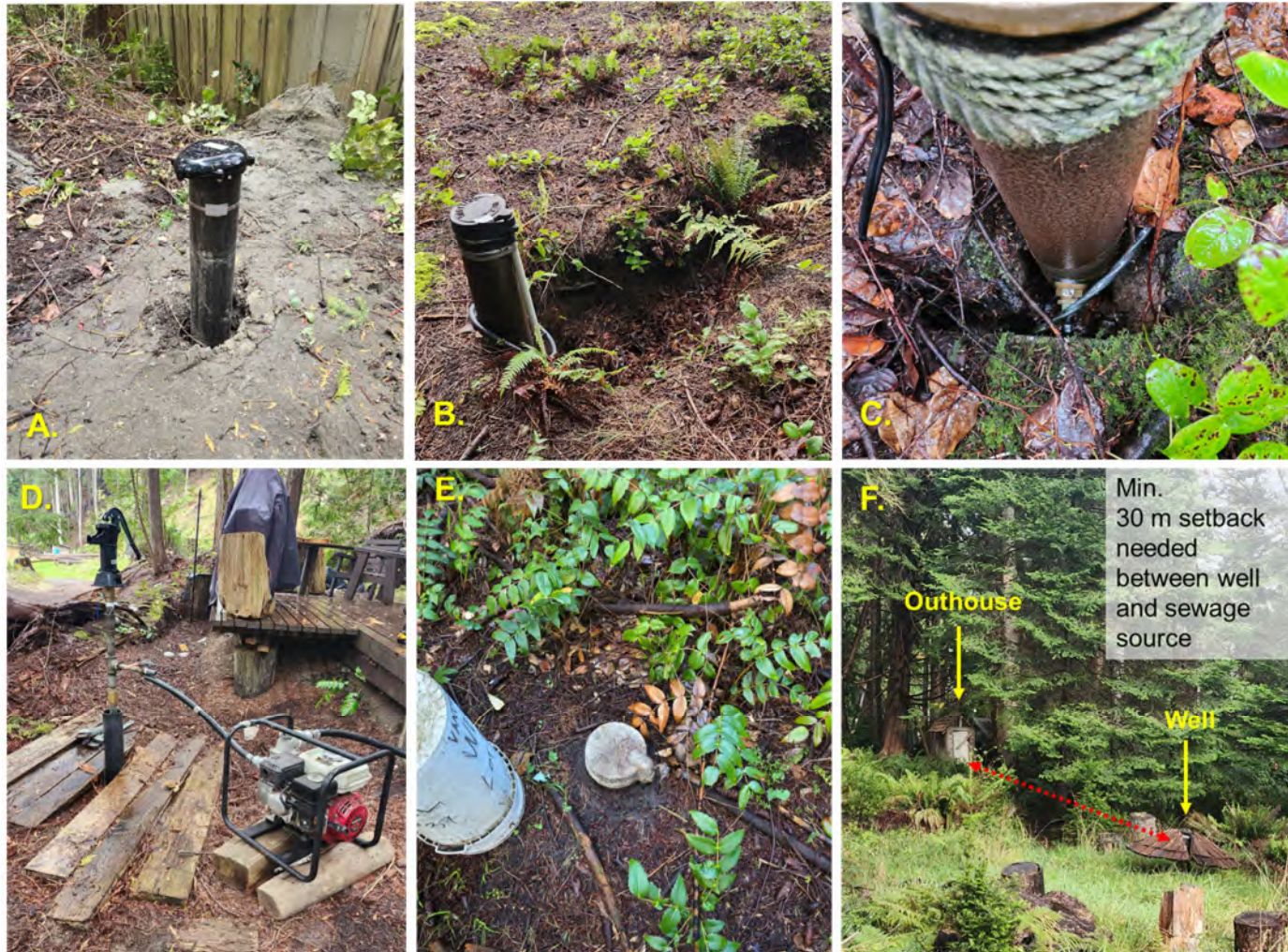
Figure 29. Savary Island well protection observations. A. New well with subsidence and unfilled annular space surrounding the casing after drilling (must be filled in with sealant and regraded). B. An unfilled trench where water lines were installed or C. annular space left open after installation of pitless adapter (water line) below ground. Both provide a preferentially pathway for contaminants to infiltrate toward the well and into the aquifer. Surface seal should be restored, trenches filled and area around well regraded to protect the well. D. Gas generator with no spill pan less than 3 m from well. An accidental spill could contaminate the well and aquifer. E. A low casing stickup (<0.3 m) increases risk of flooding, vermin or contaminant entry into a well. F. A well that is located close to a sewage source is at higher risk of contamination.
