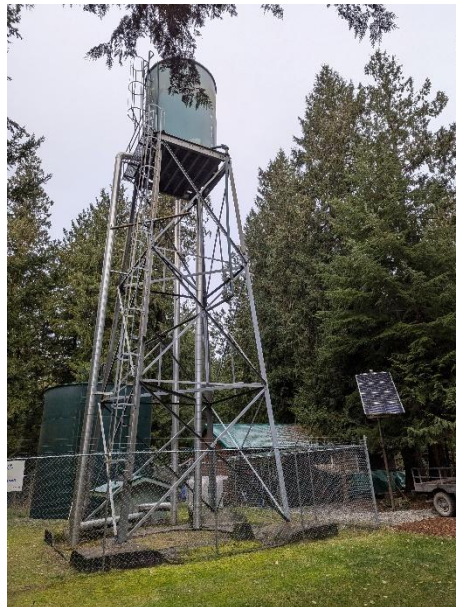
Figure 1. Existing Elevated reservoir (front) and Ground reservoir (back). Valve chamber in Between.
